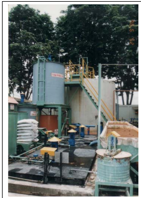
Picture 5: Waste Water Treatment Plant at P.T. Gaya Motor
